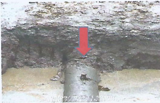
Pic1: Showing one (1no.) 2" nipple illegally installed on the pipeline
